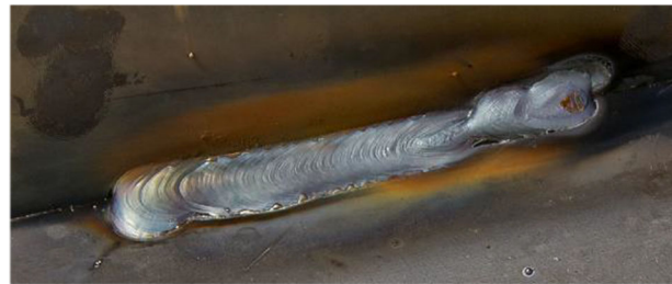
f) Colour image of a defective weld
